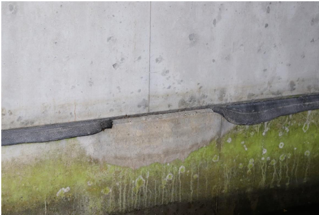
Figure 23 - South Abutment Joint Filler Loss
