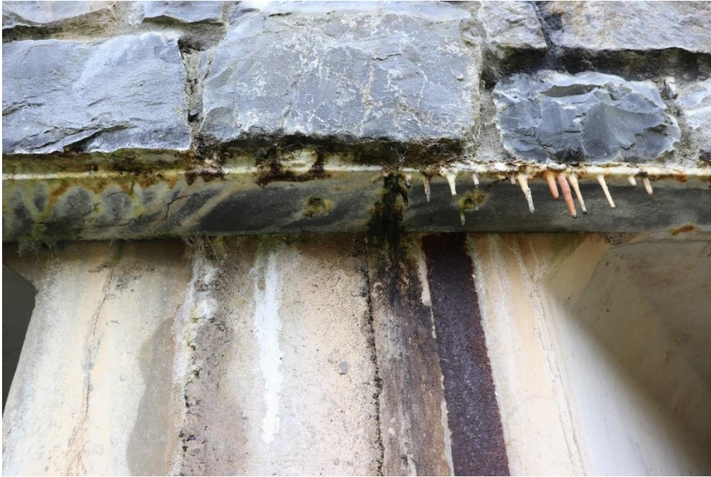
Figure 19 - Stalactites and Staining on Parapet Edge Beam
