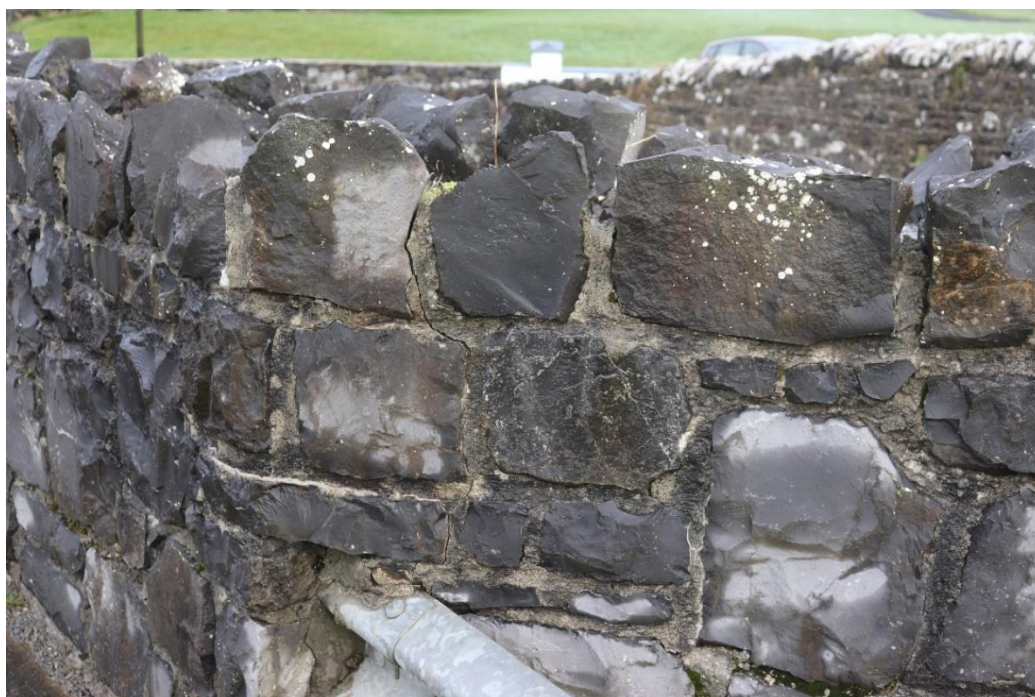
Figure 18 - Cracking of Masonry Pointing
