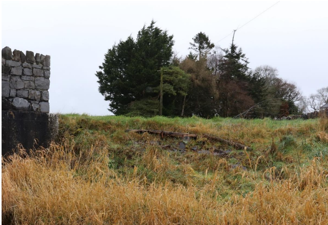
Figure 20 - Fallen Timber Post and Mesh Fence
