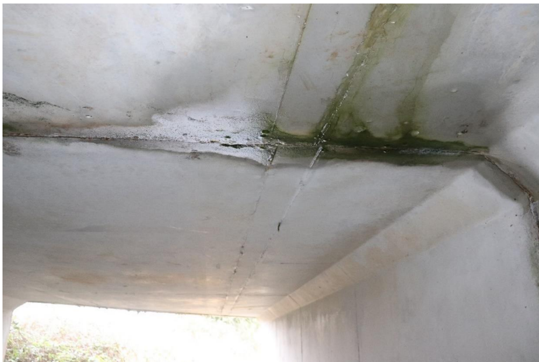
Figure 32 - Leaching and Water Seepage on Soffit of South Span
