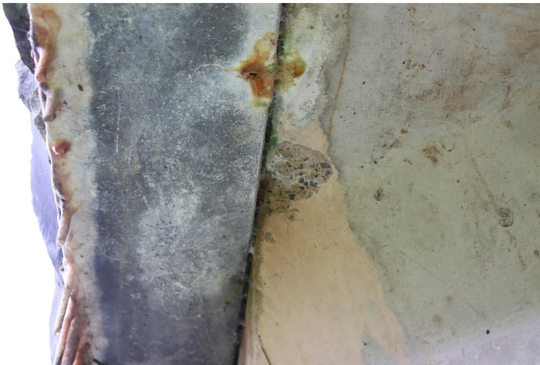
Figure 33 - Damage and Concrete Loss to Soffit of North Span
