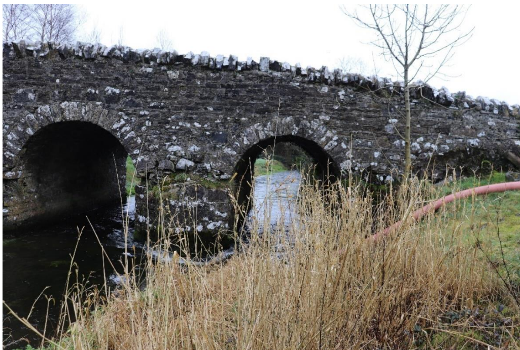
Figure 21 - Pipe on River Embankment Downstream of ST01 (Masonry Arch Bridge visible here is parallel to ST01 and not included in this inspection)
