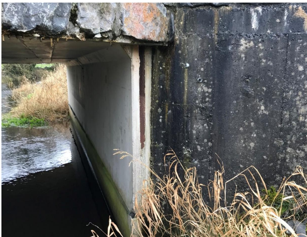
Figure 34 - Concrete Spalling around Corroded Steel Strips
