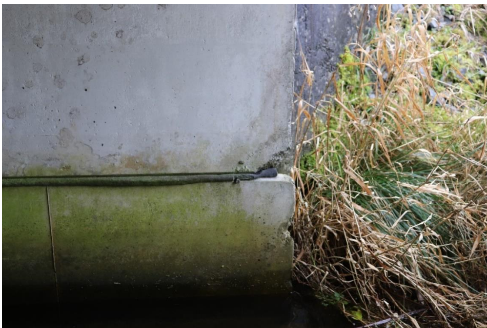
Figure 26 - Damage and Concrete Loss to North Abutment
