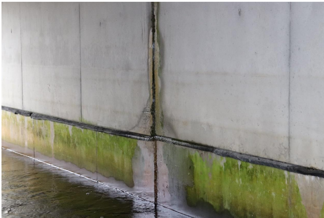
Figure 31 - Position Difference in North Pier at Vertical Joint
