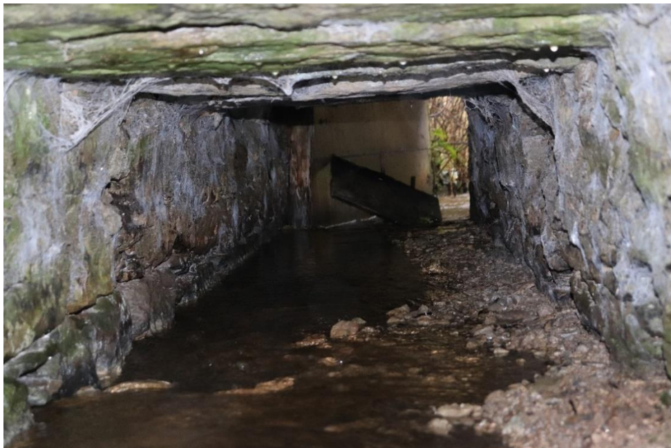
Figure 49 – Debris and Silt Build-up in Riverbed
