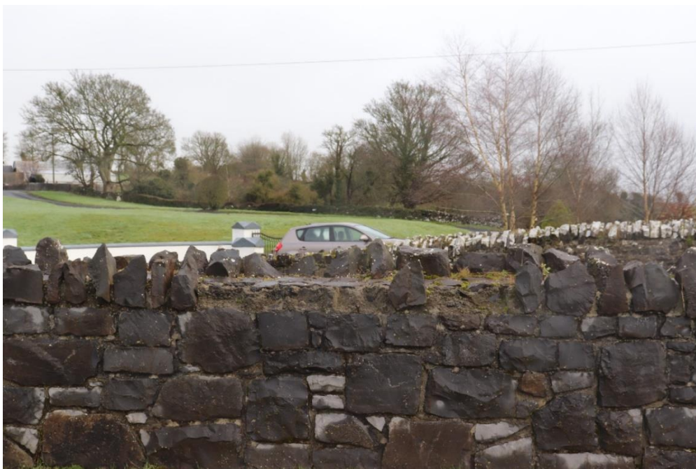
Figure 17 - Loss of Masonry Facing
