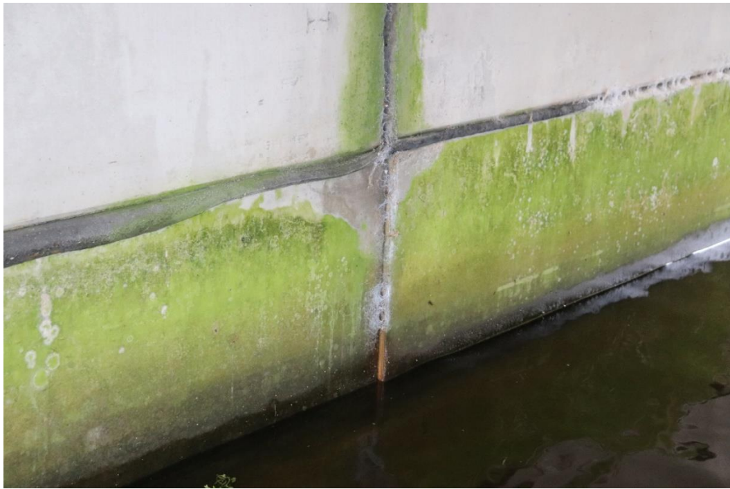
Figure 27 - Position Difference in South Abutment at Vertical Joint
