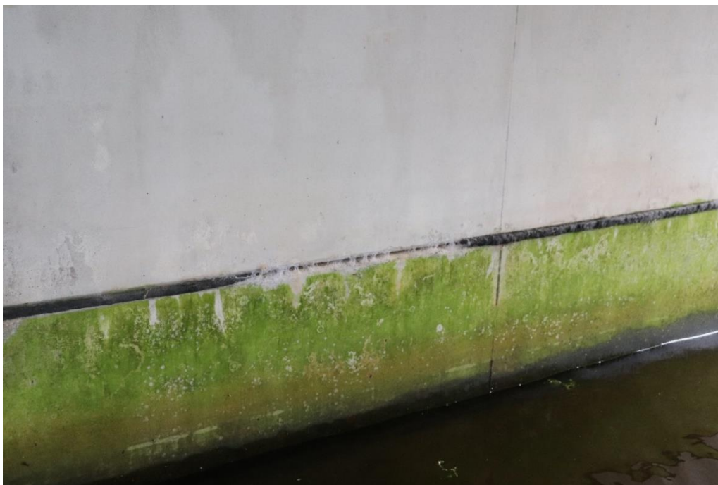
Figure 24 - South Abutment Additional Joint Filler Loss
