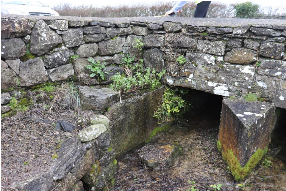
Figure 48 – Northwest Wingwall and Abutment with Vegetation Growth
