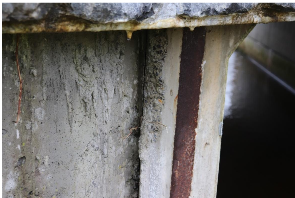
Figure 22 - Damage and Concrete Loss to South Abutment
